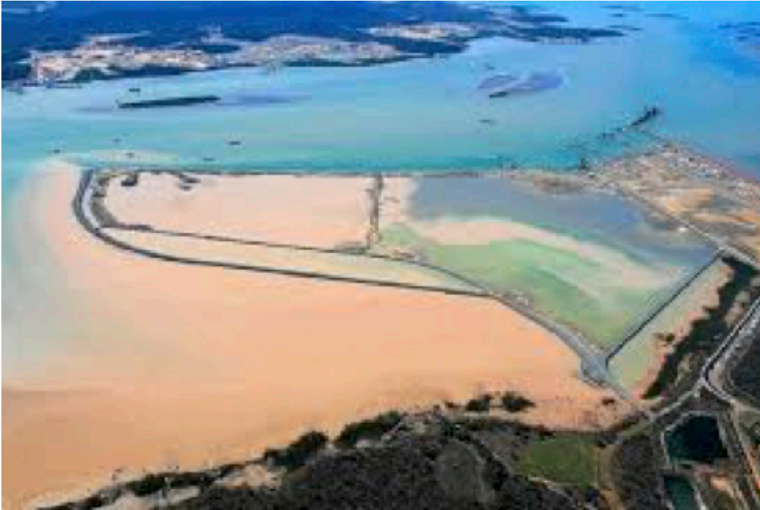
Figure 2. Dredge spoil leaking out of the bund wall in 2011. The LNG plants under construction can be glimpsed on Curtis Island on the other side of The Narrows.
