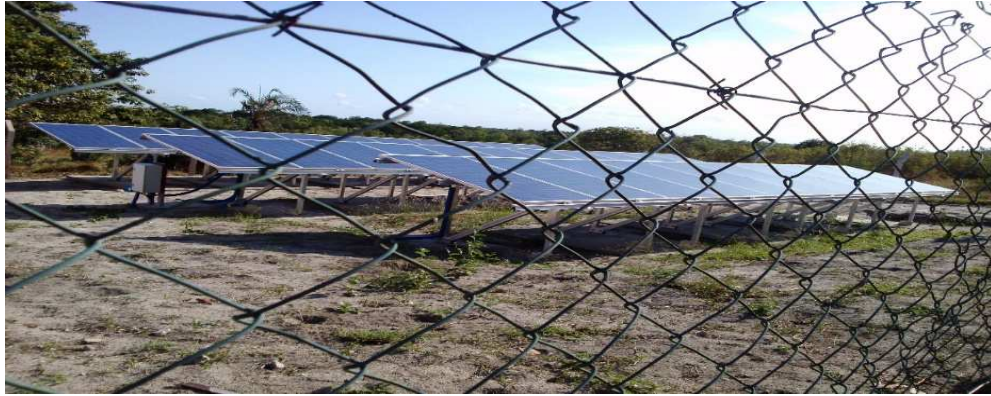
Plate 2. Solar Panels Installed in Kisiju-Pwani to constitute a min grid plant
