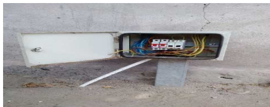
Plate 7: The connection box which was hit by the motor bike.
