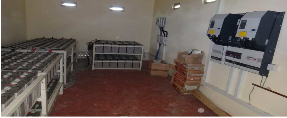
Plate 4: The batteries, DC side switch gears and protection, charger controller, inverter, AC side switch gears and protection installed in a power house
