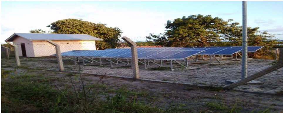
Plate 3: A complete setup of the min grid with solar panels and the Battery bank house
