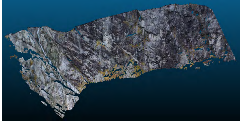
FIGURE 5.6: Point cloud of a cliff. This was imaged from roughly 200 meters away. The cliff is 50 m high. This point cloud show great detail.
