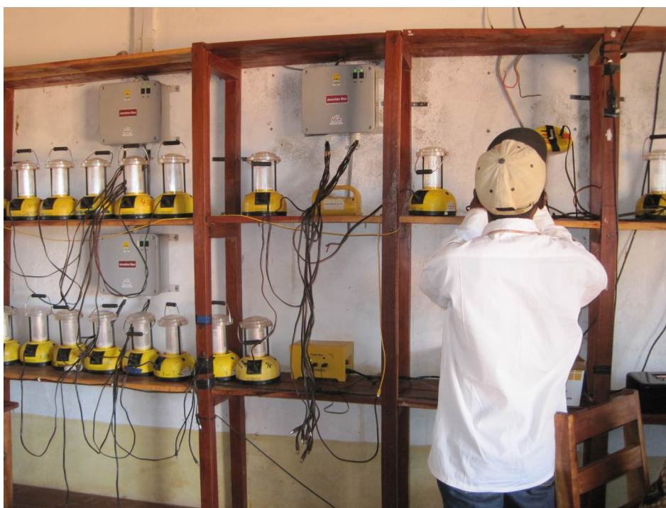
Illustration 3: The lantern and phone charging room. Photo: Author.
