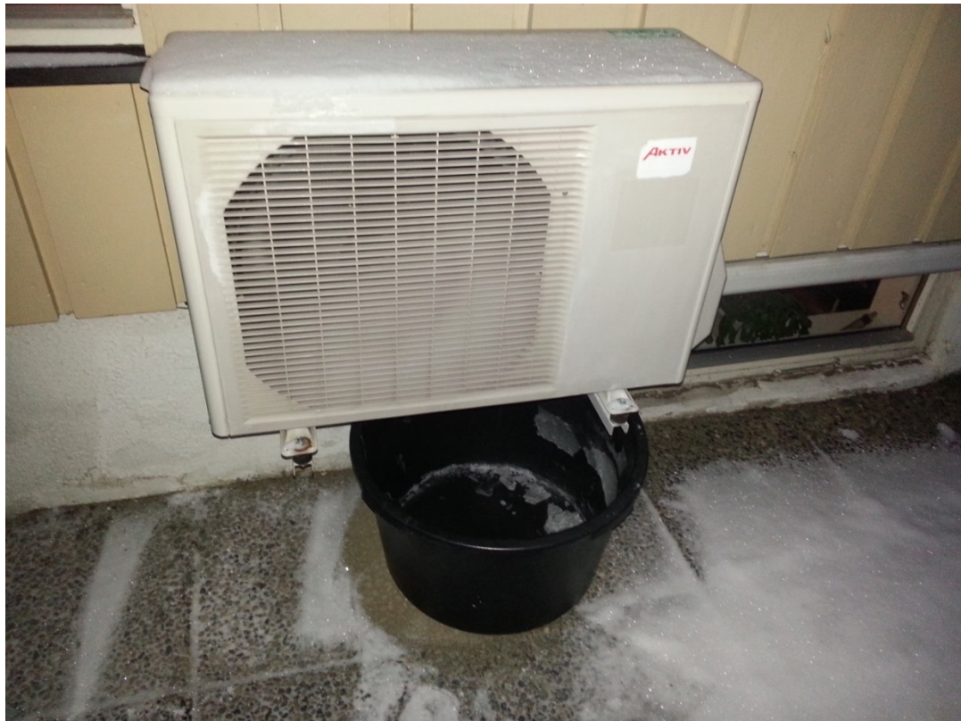
Figure 3. Bucket household #6 used to collect water run-off from heat pump defrost cycle.
