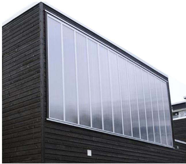
Figure 4.5: Solar collector on south wall of House A at Rudshagen.
