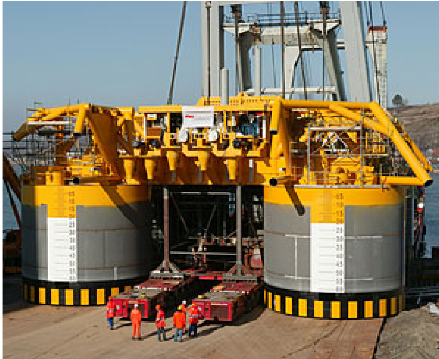
Fig 51 Dimensions of the sub-sea well template for eight wells with control equipment ©Hydro/ Ormen Lange project homepage
