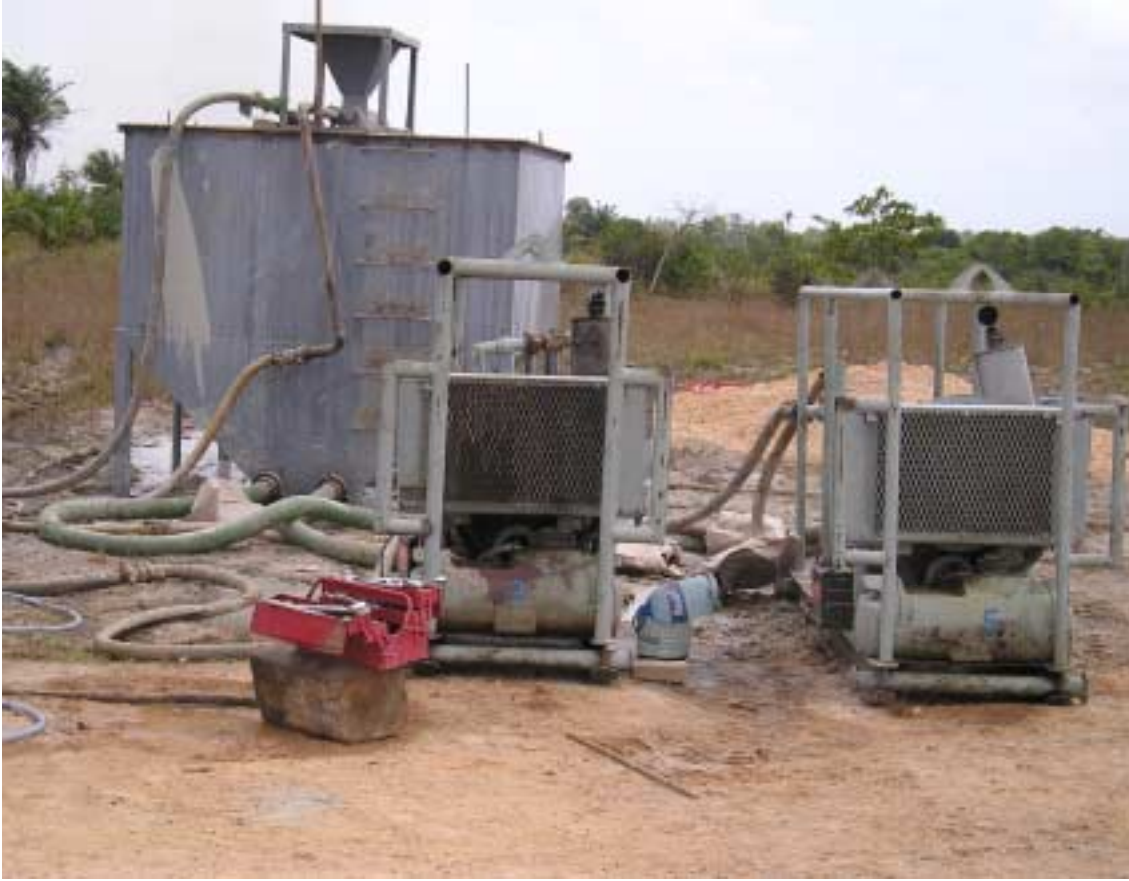
Figure 3.5: Depicts the mixing tank and mud pumps at Kimbiji site. The pumps used to pump the mud from the mixing tank to the cyclones before pumped again to the borehole.
