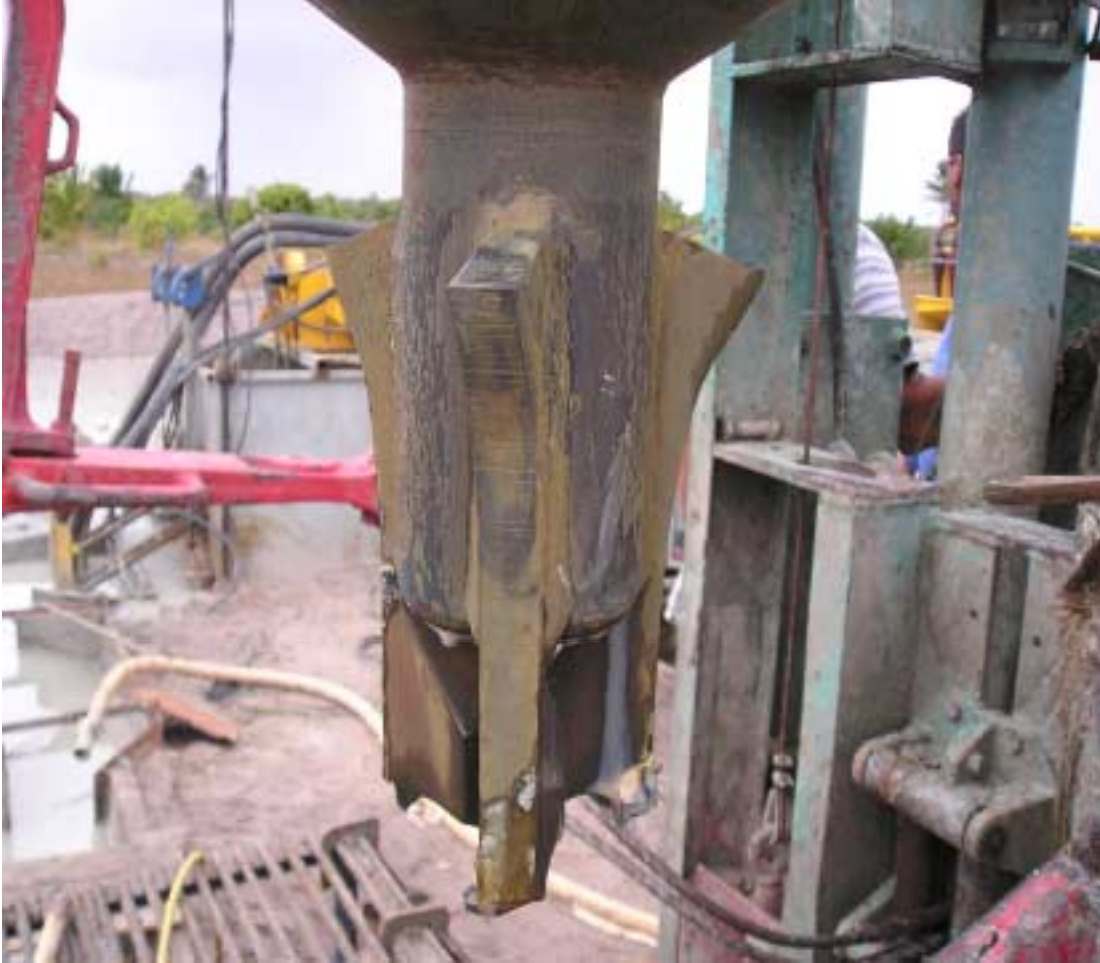
Figure 3.3: Worn drag bit as it was pulled out from the well at Kimbiji site
