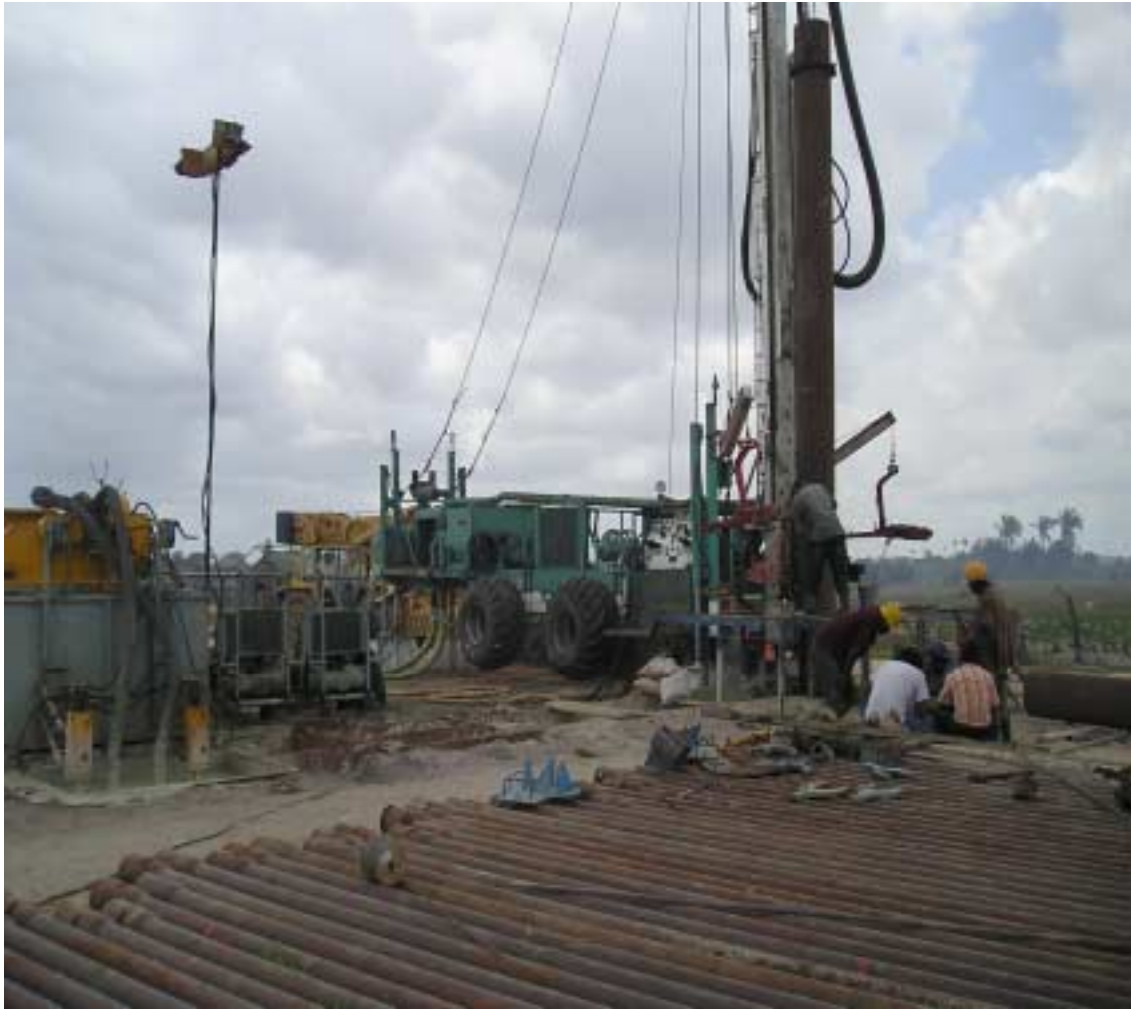
Figure 3.1: Depicts the drilling rig to the right, drill pipes, mud pump and settling pit in the left at Kimbiji site
