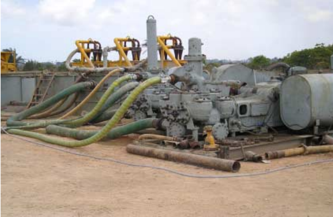
Figure 3.6: Mud pumps at Kimbiji site. These mud pumps (right) used to pump the mud from settling pit (left) to the borehole.
