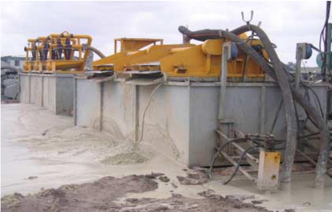
Figure 3.4: Depicts mud pit, shaker, and cyclones at Kimbiji site. The shaker used to separate sand, silt and other cutting materials from the mud coming direct from the borehole for further circulation.
